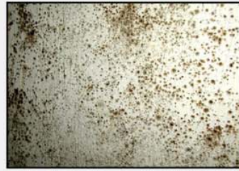
Unightly stain caused by mold and mildew.
